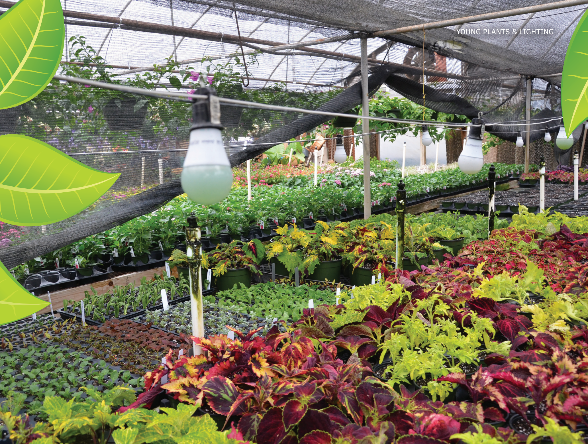
Figure 1. Non-horticultural LED lamps installed in this greenhouse have filled up with water.
